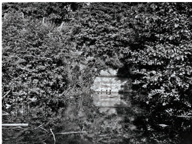
The bricked-up west portal in 1963; a few years before the cutting here was backfilled with spoil. Photo Richard Amott
